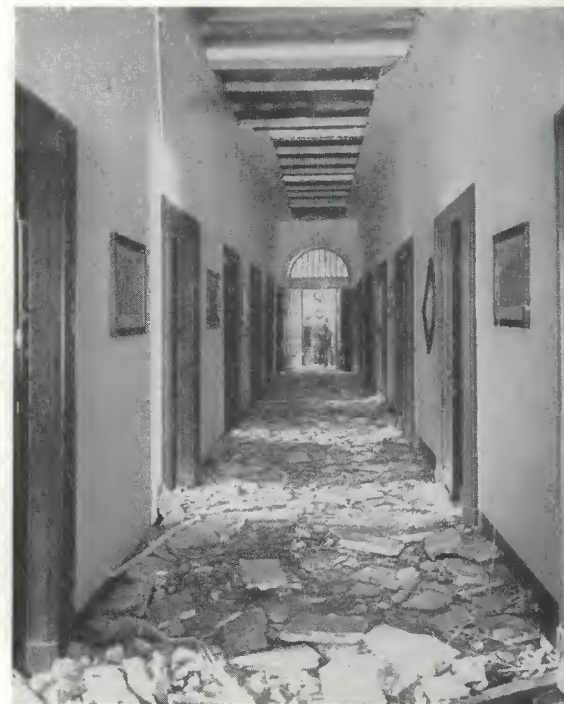
One of the corridors in the Governor's Palace showing damage from bomb blast.
