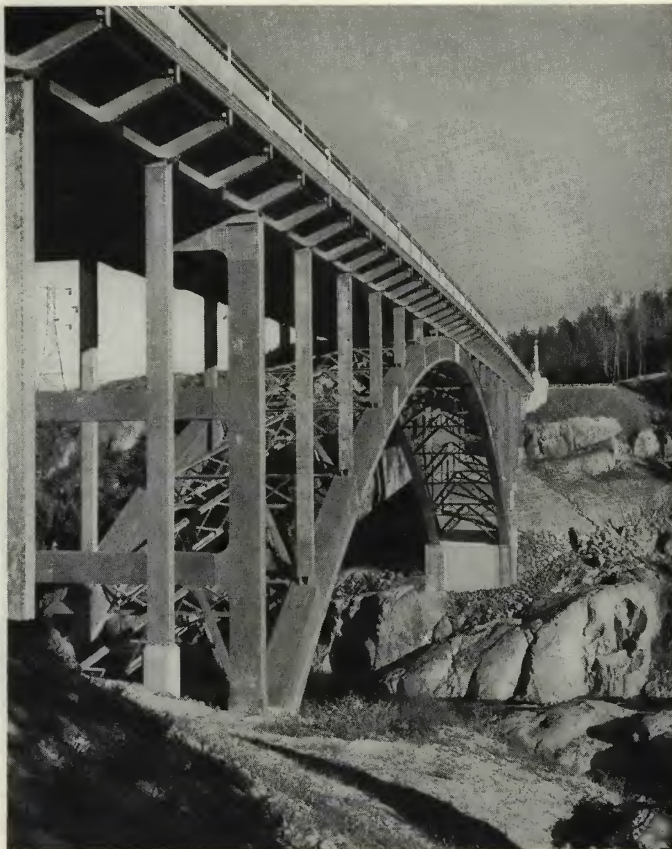
First all-aluminum bridge in the world — Arvida (Quebec) Canada Photo courtesy Aluminum Co. of Canada, Ltd.
