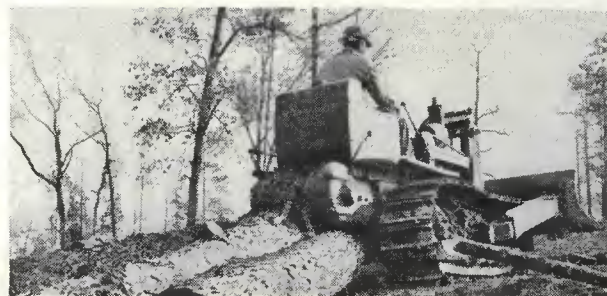
Snaking logs! Plenty of hefty pull for moving timber with a rear-mounted winch on the TD-6.
