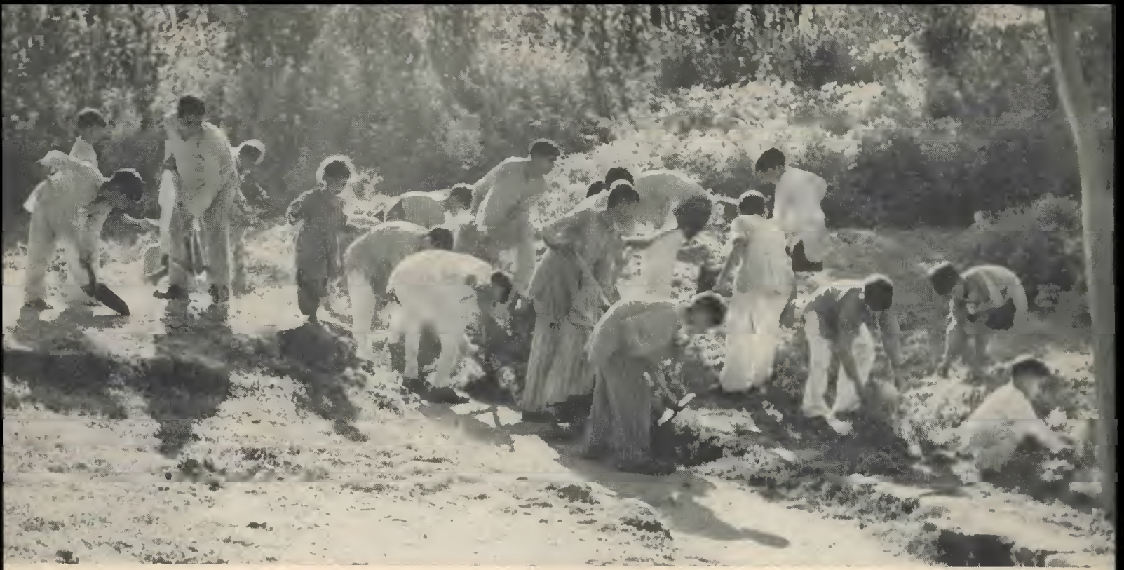
School children leveling the ground for road construction. Dhansal community project in Jammu.
