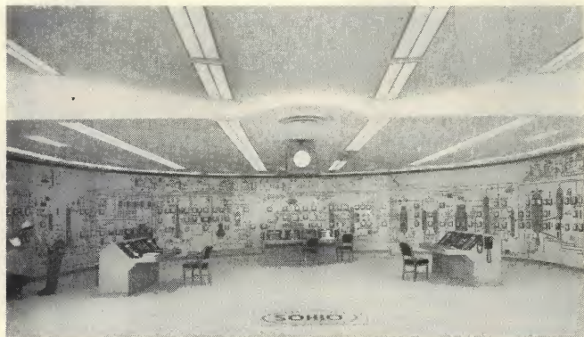
Control room at SOHIO's Toledo refinery, where all operations of this huge project are controlled and recorded. Complex instrumentation such as this is a major phase of Kellogg's complete engineering, procurement, and construction service to the petroleum and other process industries.
