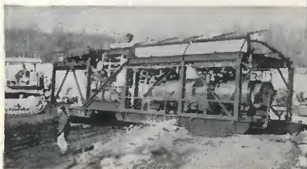
Section of plant on way to site. Premature melting of snow in places required dragging of unit on dirt roads. Note integral runners.
