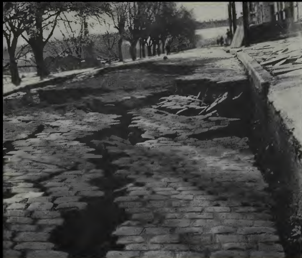
Earth tremors destroyed these riverside streets in Valdivia.
