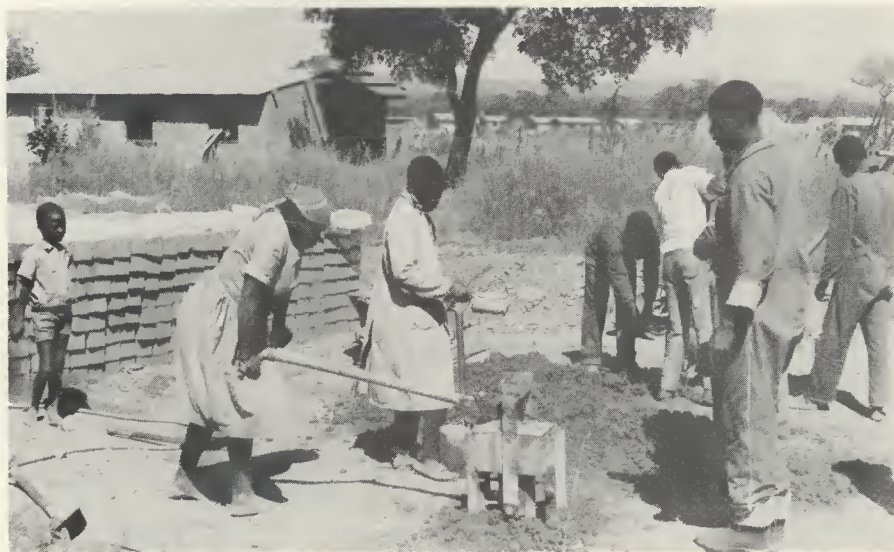
Zambians pressing the earth and cement mixture to produce the bricks for a house in Kafue's self-help squatter upgrading project.
