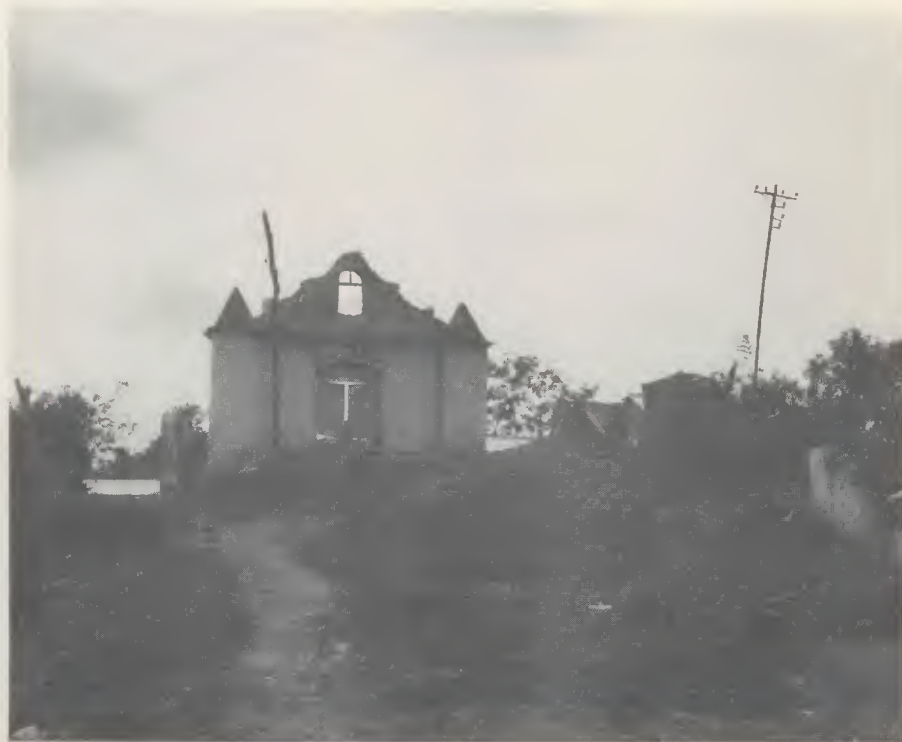
Only the front facade of the Roman Catholic Church survived the earthquake. Even the front door remained padlocked although there is nothing behind the wall, which now stands like a monument on a hill overlooking the town.
