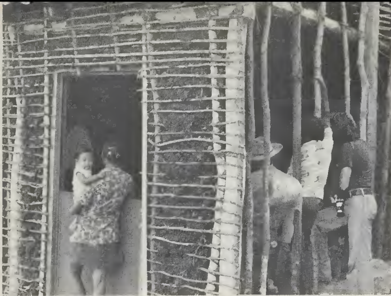
A bajareque under construction shows the building technique which was most successful in withstanding the earth tremors. The bajareque, however, is considered undesirable by status-conscious El Progresans.
