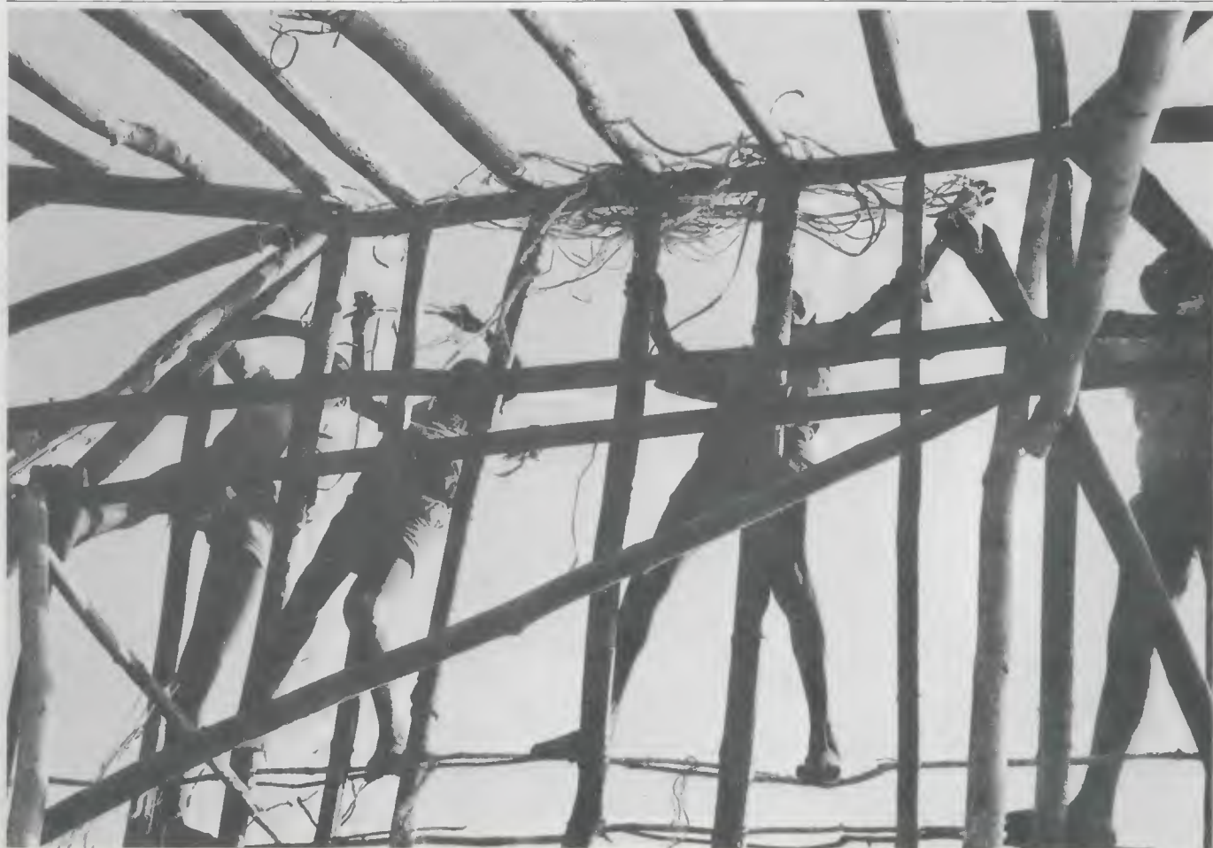
some of the older boys help put a roof on the new house for the teacher
